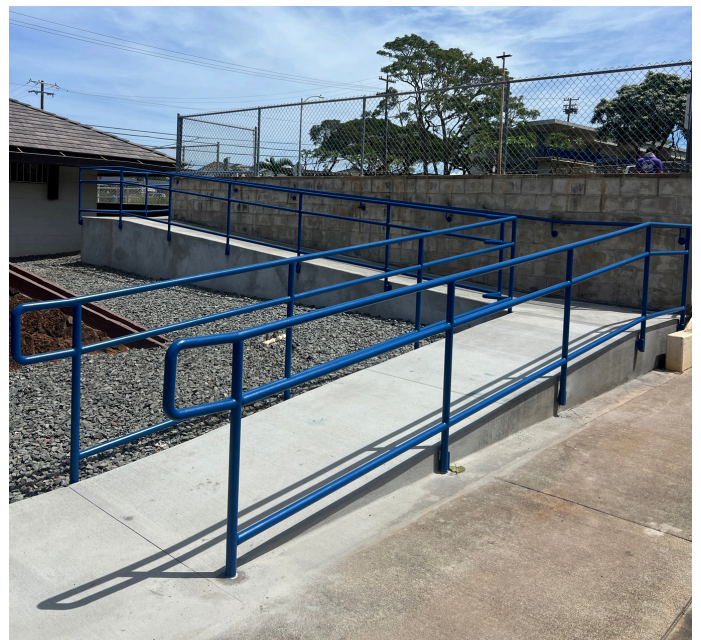
Completed ramp from the upper parking lot to the Ozawa Hall and temple.
